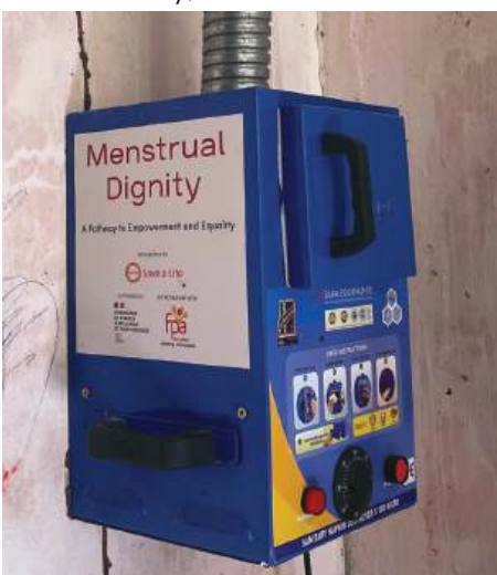
Sanitary Pad Incinerator
